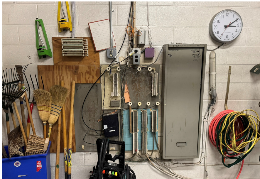
Telephone system demarcation point in boiler room
