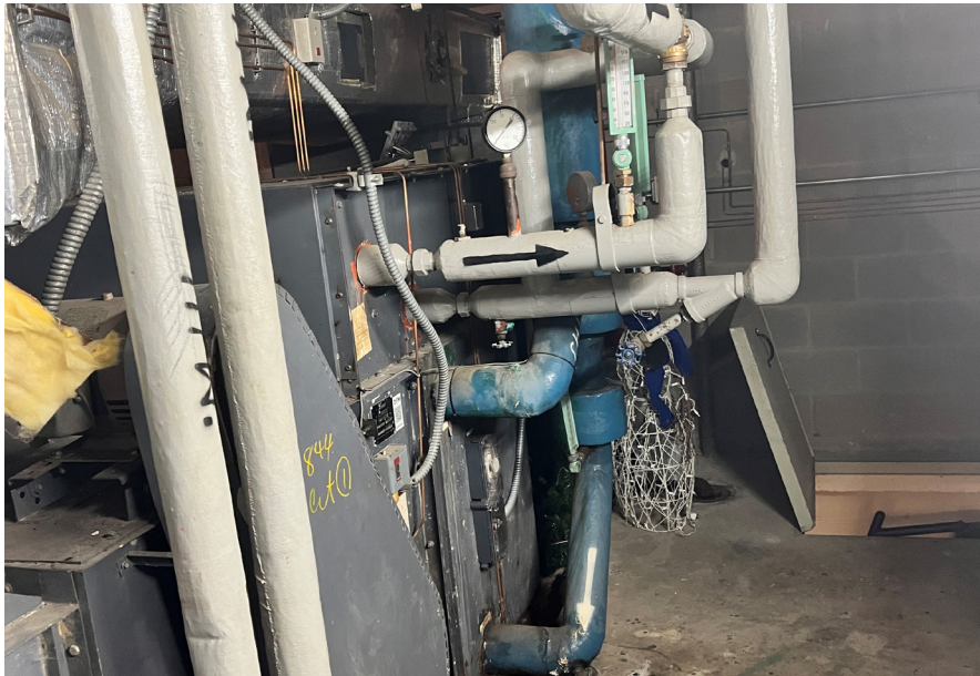
Existing air handling unit for classroom and media center areas
