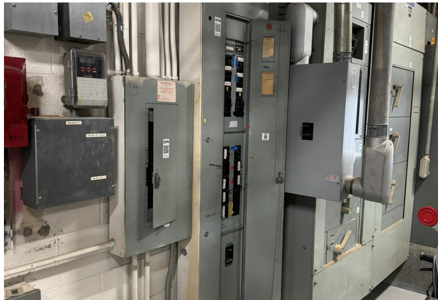
Enclosed circuit breaker and tap serving gym addition
