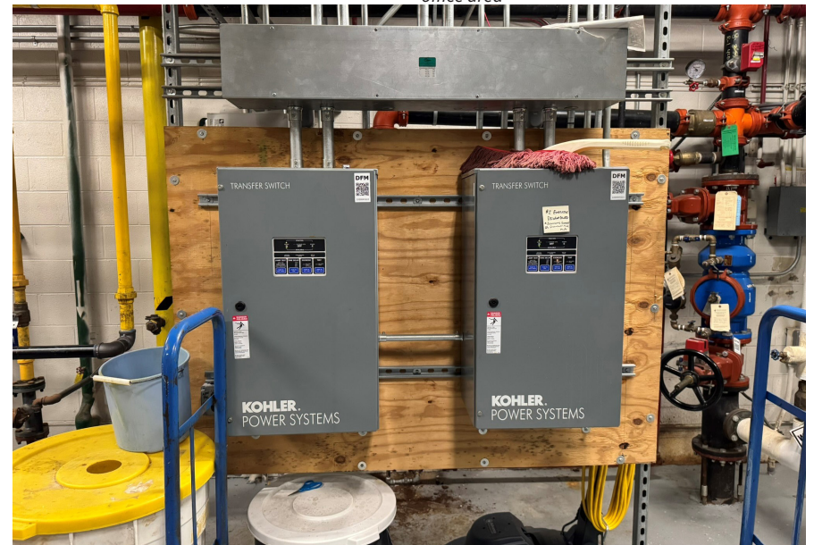
Automatic transfer switches in boiler room
