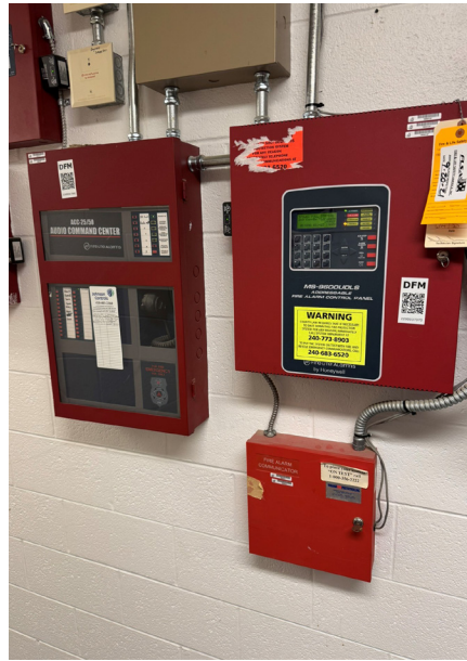
Fire alarm control panel and voice control panel
