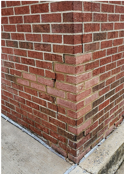
Deterioration on Service Enclosure
