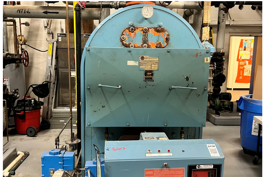
Existing heater water boiler
