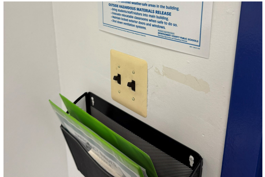
Typical classroom lighting controls
