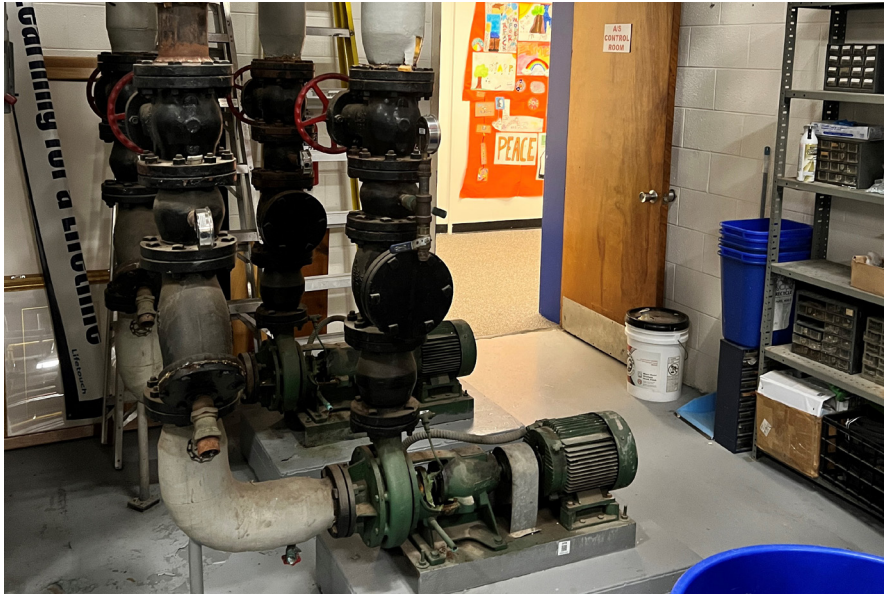
Existing heating water pumps
