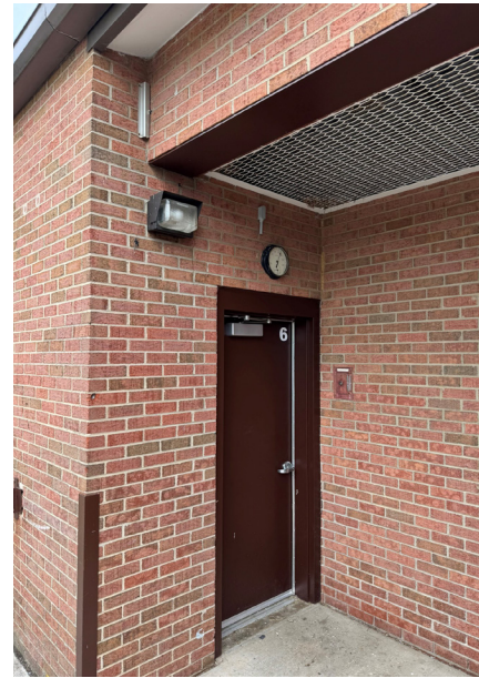
Exterior, wall pack lighting fixture
