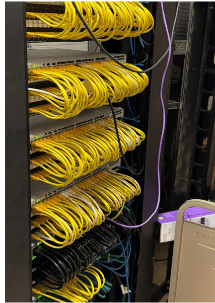
Data racks in storage room
