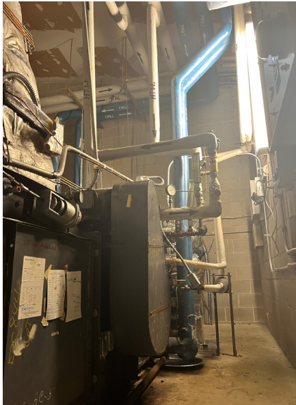
Existing air handling unit for admin/health suite
