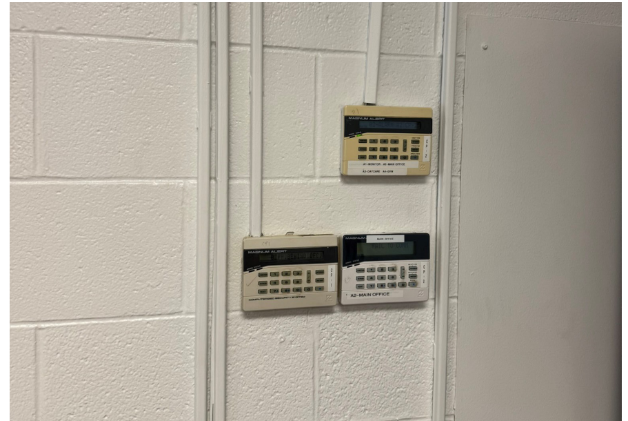
Intrusion detection system keypads
