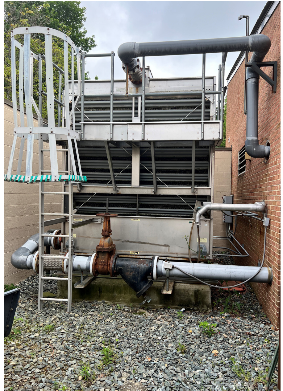
Existing cooling tower
