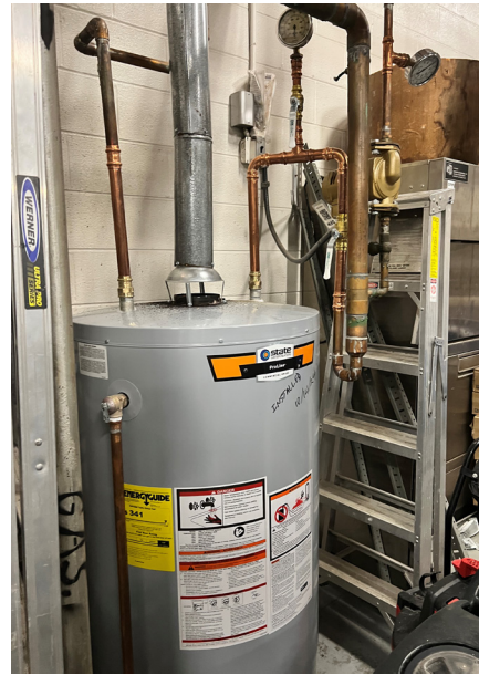
Domestic water heater and hot water circulation pump
