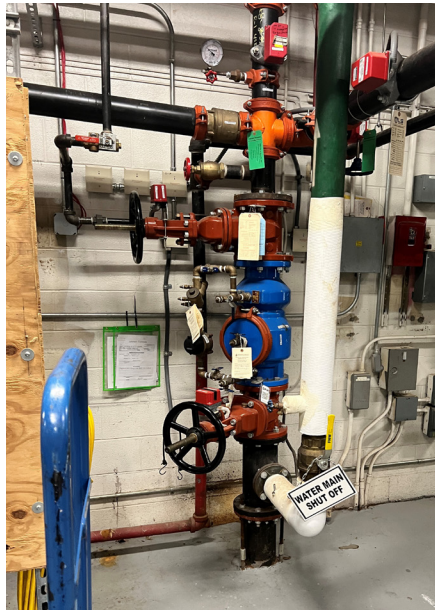
Combination fire and water and sprinkler backflow preventer
