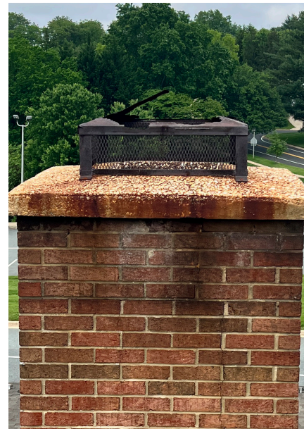
Deterioration of Chimney Cap
