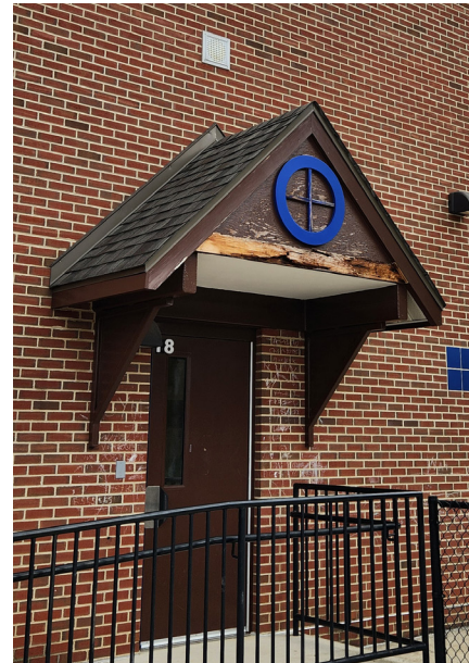
Deterioration on Gym Facade
