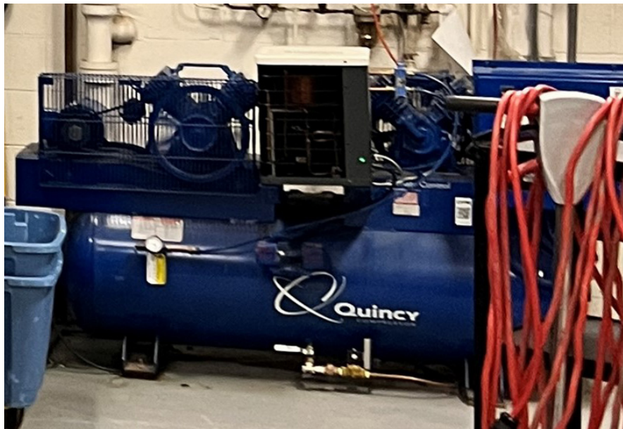
Existing boiler room air compressor
