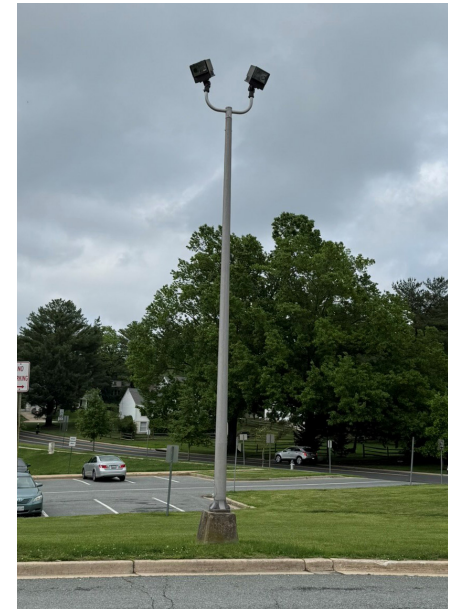
Exterior, pole-mounted lighting fixture
