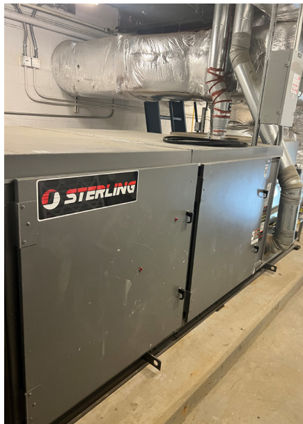
Existing gymnasium H&V unit
