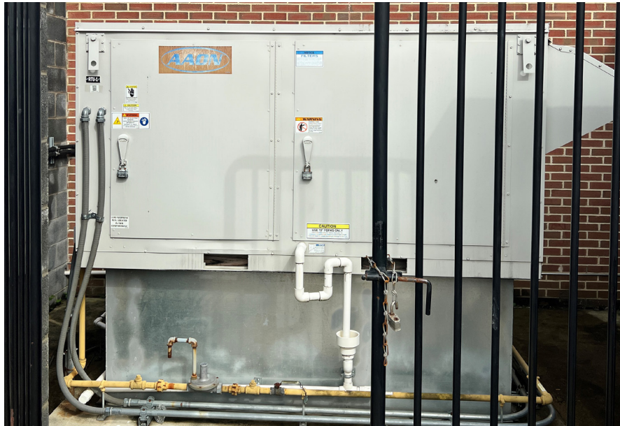
Existing gymnasium lobby rooftop unit
