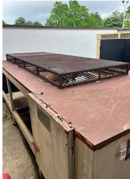
Existing condensing unit for admin/health suite
