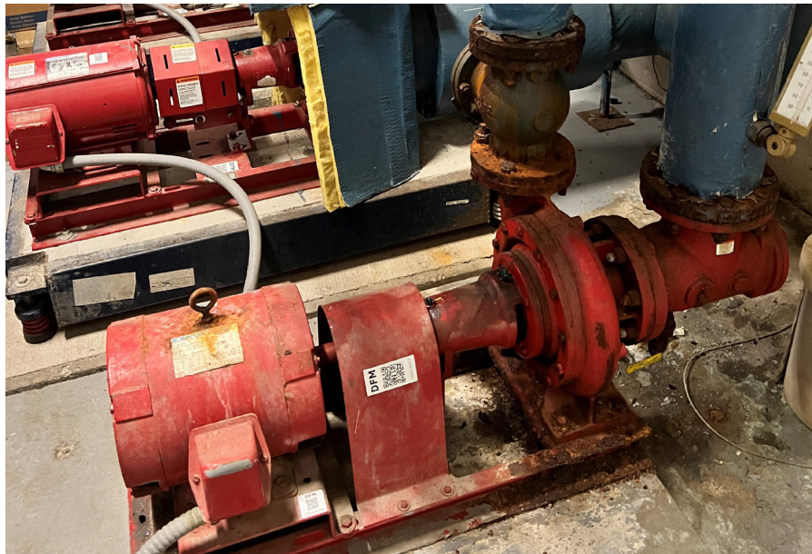
Existing heater water pumps
