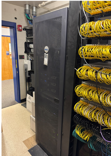
Data racks in storage room
