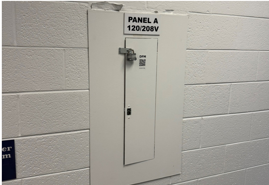
Typical branch circuit panelboards in corridor
