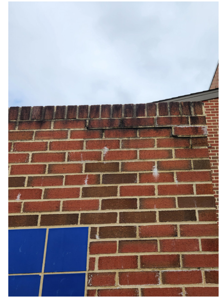
Deterioration on Mechanical Enclosure
