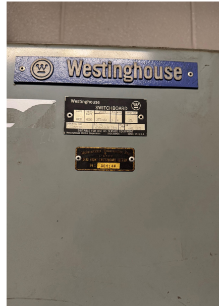
Switchboard nameplate inconsistency
